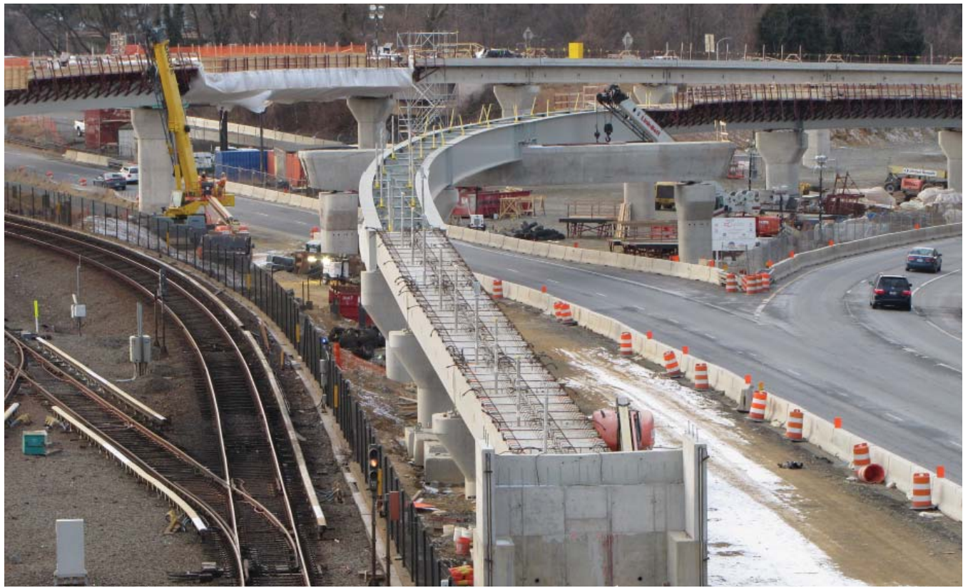
Junction of the Project with the Existing Metrorail Orange Line Image courtesy of MWAA
