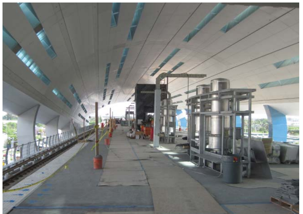
Installation of the Miami International Airport station - platform level equipment (windscreen with bench, signage supports, elevator, etc.) Image courtesy of MDT
